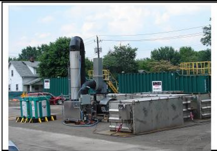
Figure 1.4 Thermal Treatment Unit for Oily Wastes
